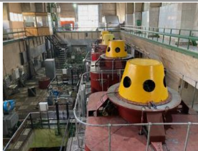
Photo 8: Pamir-1 HPP powerhouse
