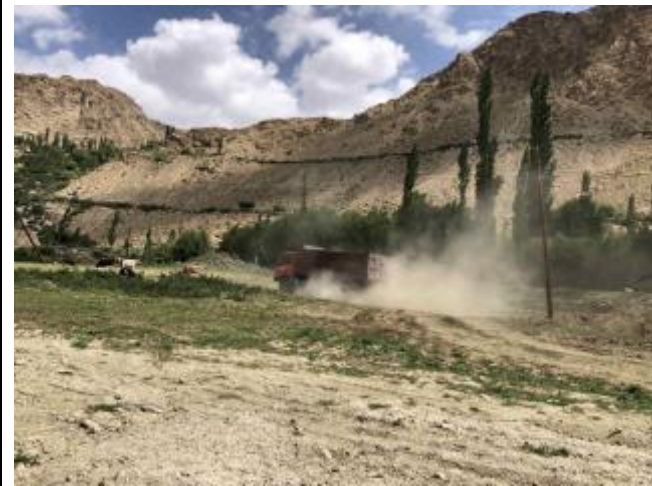
Photo 35: Construction traffic dust at intake
